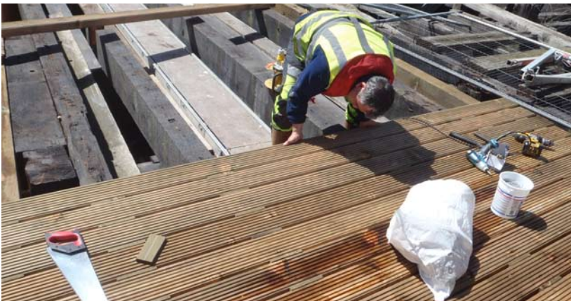
ALL DECKED OUT/ THE SWING BRIDGE IS CURRENTLY HAVING THE DECKING REPAIRED ON THE WEST WING AND IS DUE TO BE BACK IN FULL OPERATION IN OCTOBER
