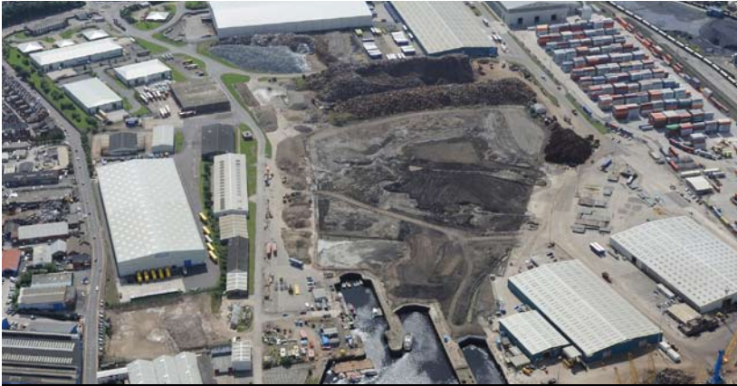
GET YOUR FILL/ TO DATE WE HAVE FILLED TYNE DOCK WITH 108,000 CUBIC METRES OF SOIL AND CLAY – ONLY 32,000 CUBIC METRES TO GO!
